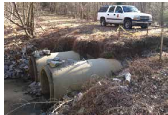
Washed out culverts in Beddingfield Creek on Clemmons Educational State Forest, Jan. 2014. We are seeking grant funds to restore this stream section and install a better crossing.
